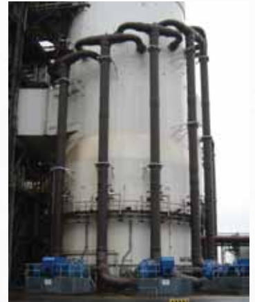
Power Station Absorber
